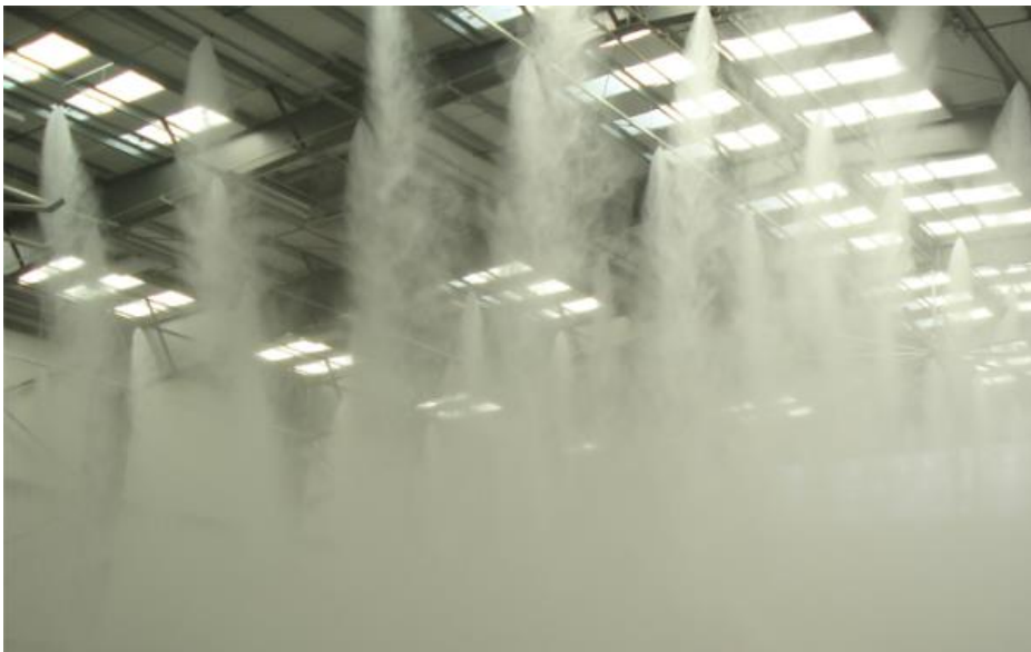
Water Mist Suppression System
