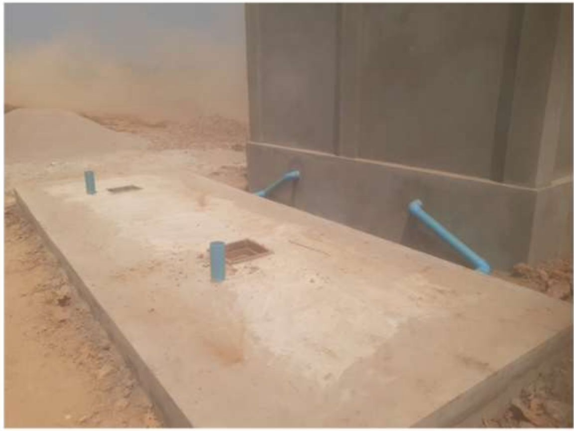
2 Units Latrine to Septic Tank Wrong Connection
