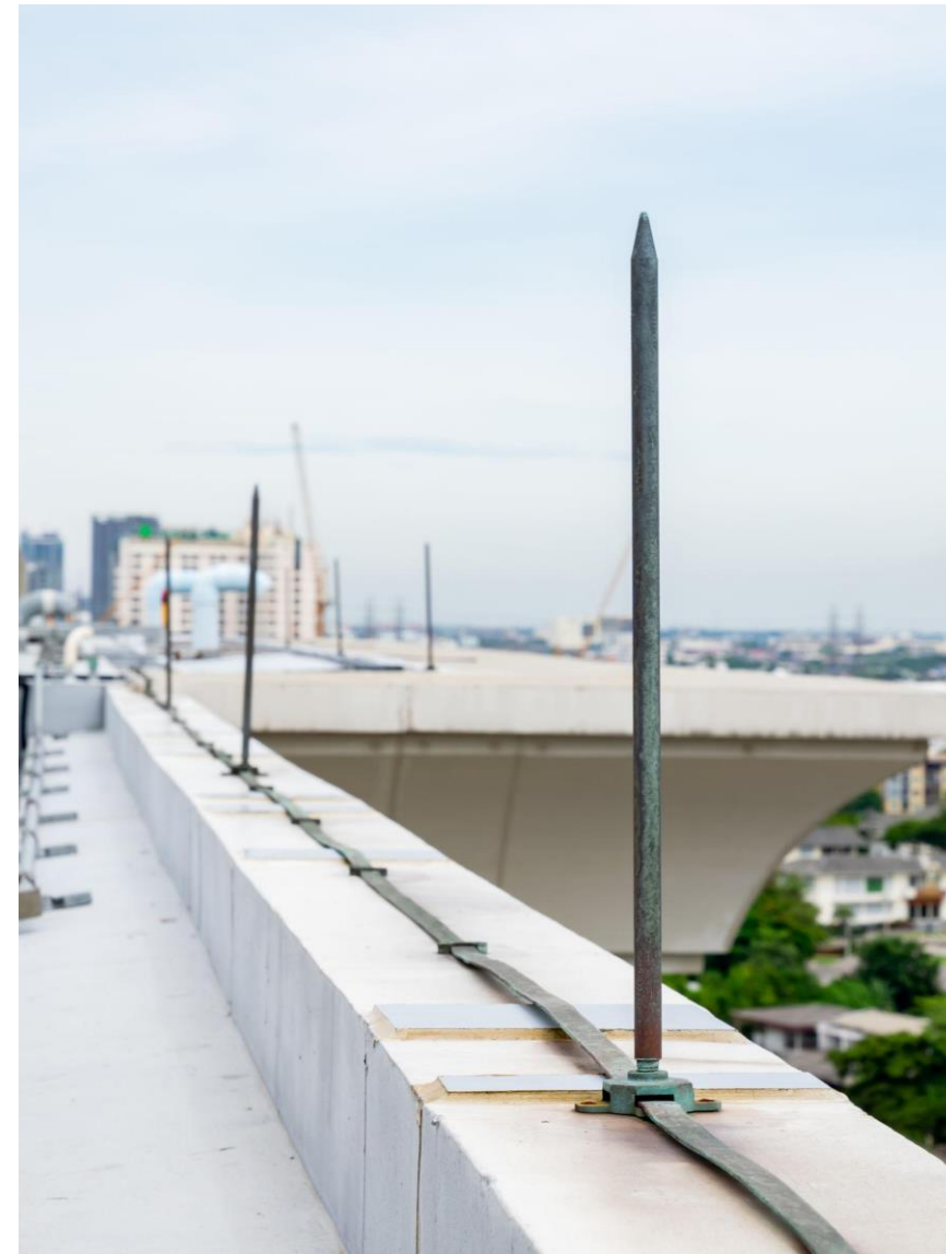
A lightning protection system is installed on the roof of a high-rise building as a bolt of conductor lightning to the ground, ground rod on the sky background.
