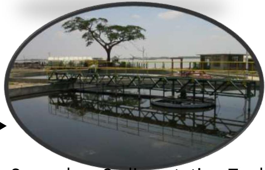
• Secondary Sedimentation Tank
