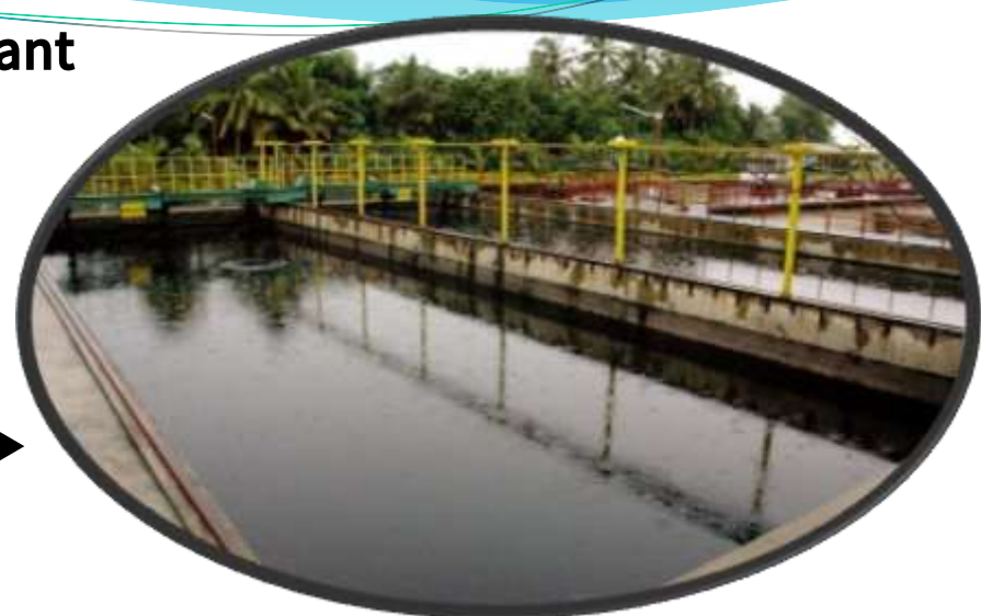
• Primary Sedimentation Tank
