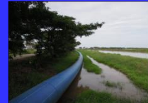
Transmission pipeline from Nyaungnapin
