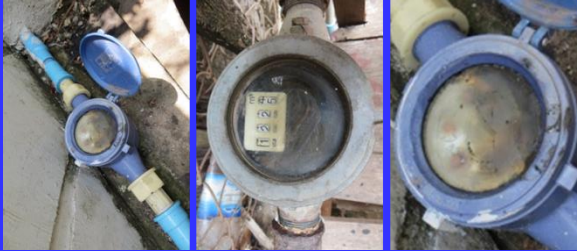
Damaged meters without meter Accuracy
