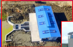
Intake Pumping Station
