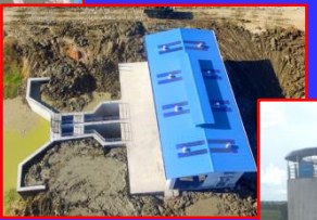
Intake Pumping Station
