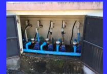
Housing booster pump
