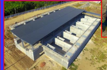
Rapid Sand Filter Basin
