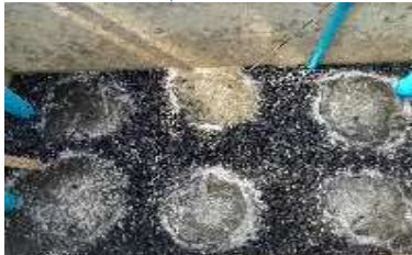
Moving Bed Bio-rector Tank (Nitrification)
