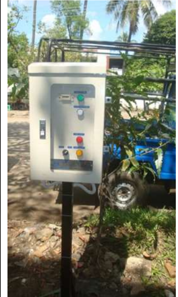
Level Control system Type-B
