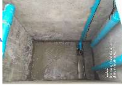
Sludge Holding Tank
