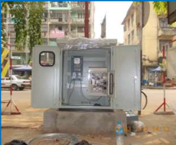
Control Panel Board
