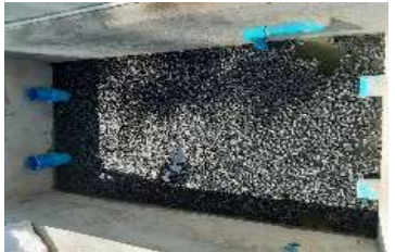
Moving Bed Bio-rector Tank(BOD Removal)
