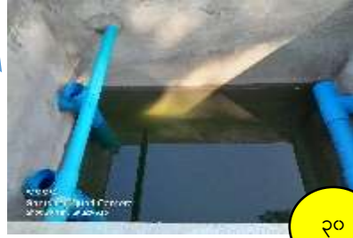
Secondary Sedimentation Tank
