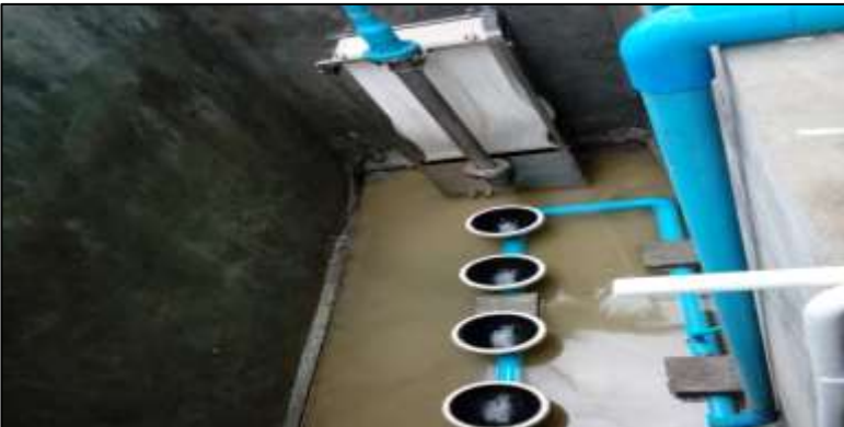
YCDC Office Housing Compound (30m 3 /day)
