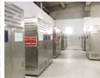
11/.4kV, 2MVA, Drytype X'mer, HUYU
