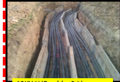
12KV U/G cable, 2 Lines Universal
