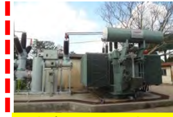
66/11kV, 35MVA X'mer HUYU, China
