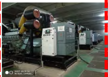
11kV Output, 2MVA Gensets x 6 No, Mitsubishi
