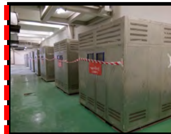
11/.4kV, 2MVA, Drytype X'mer, HUYU
