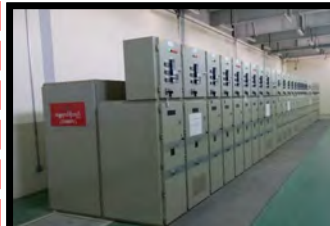
12kV Switchgears,(Type Test) Siemen, SIMOPRIME Hainam, Vietnam
