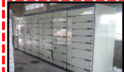
400V MSB. Blockset (Type Test) Schneider. Hainam
