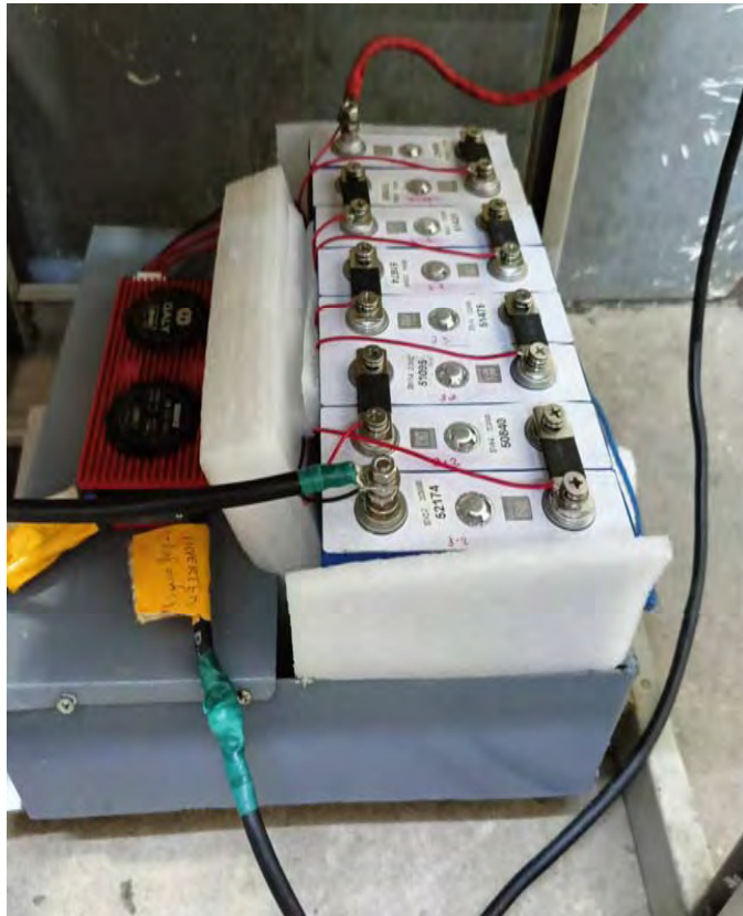
LiFePo4 battery with Daly BMS control unit
