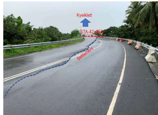
Differential settlement along the roadway
