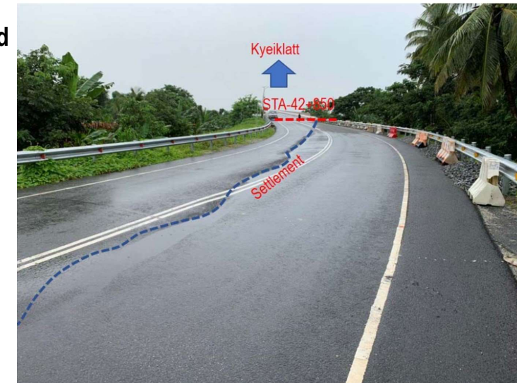
Differential settlement along the roadway
