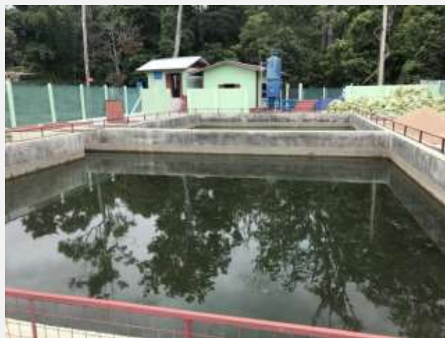
Operation of WTP at Nar Yaung Spring
