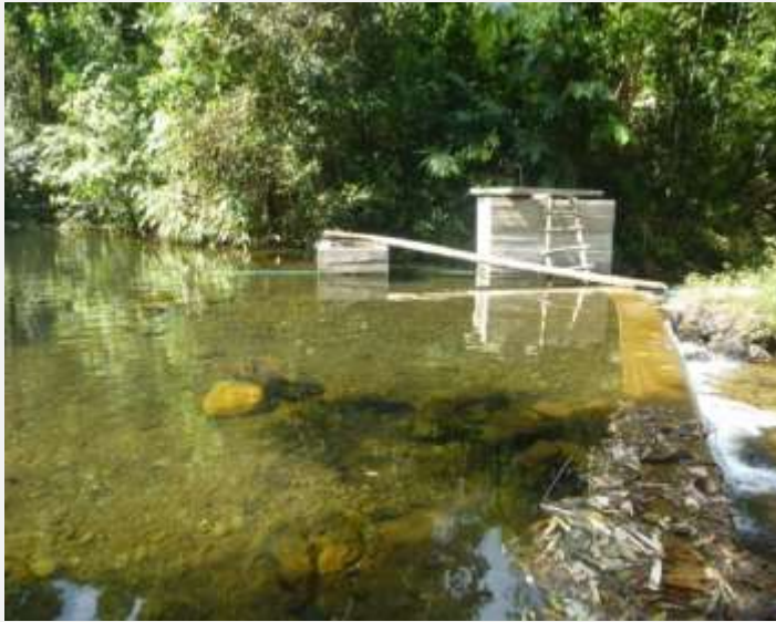
2 nd Intake Facility
