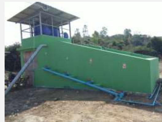
Alum dosing House and Aerator
