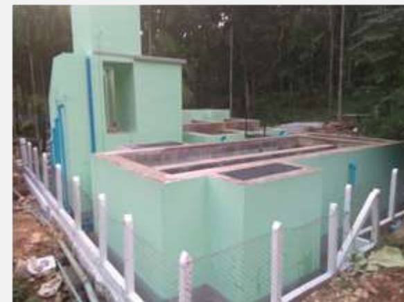
Slow Sand Filtration Facility
