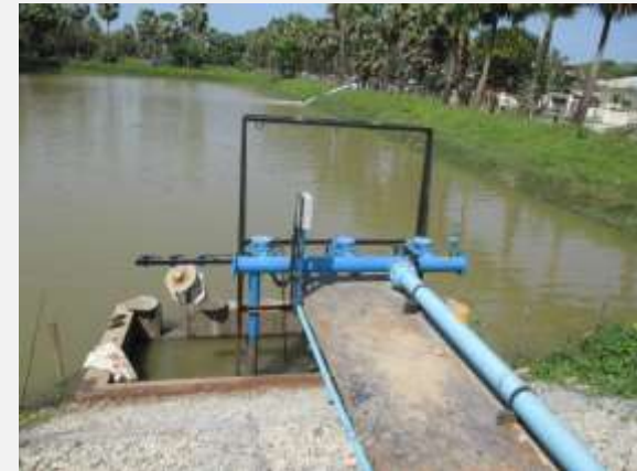
Storage Pond and Pump
