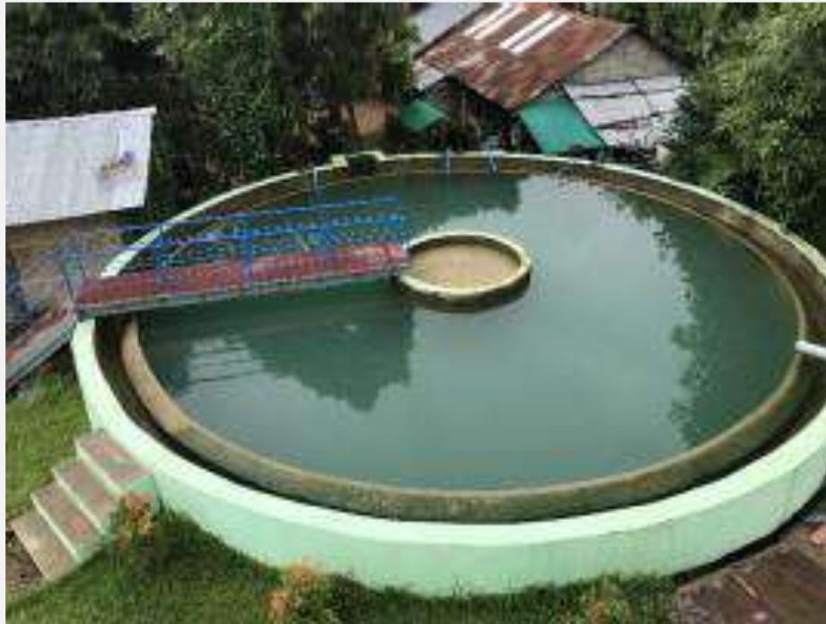
Operation of Clarifier
