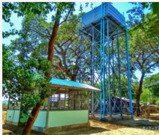
Elevated Tank at Nat Lu Htaik Pan Quarter
