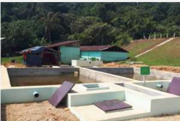
Slow Sand Filtration Facility
