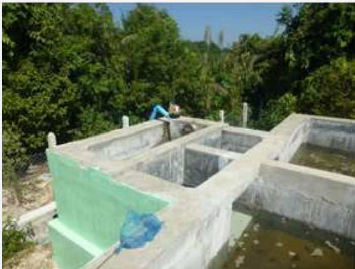
Slow Sand Filter Facility
