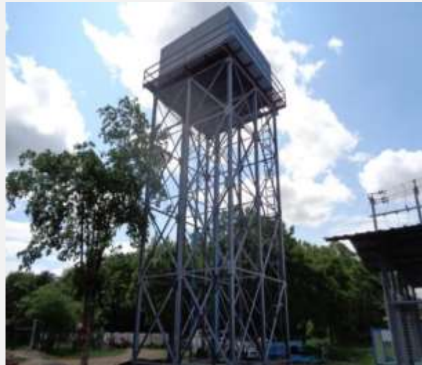
Elevated Tank at Than Lar Quarter
