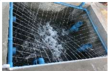
Primary Sedimentation Tank
