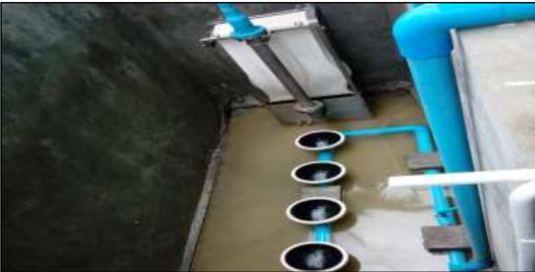
YCDC Office Housing Compound (30m 3 /day)
